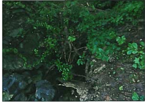
D-NS-10: Erosion observed downstream of the outfall
