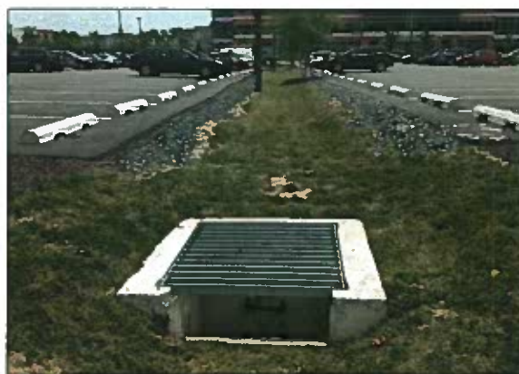
R-SWM0424: Dry swale with filter strips that capture the parking lot runoff on Millennium Drive
